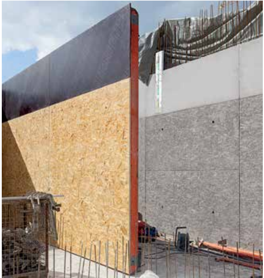
With TRIO Structure, SB 3 architectural concrete requirements are fully met. The OSB sheets and FinPly formlining were neatly screwed on at the rear.
