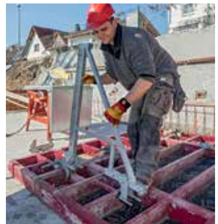
The working platforms are mounted on the element of the corresponding width and also remain attached to the formwork during temporary storage.
